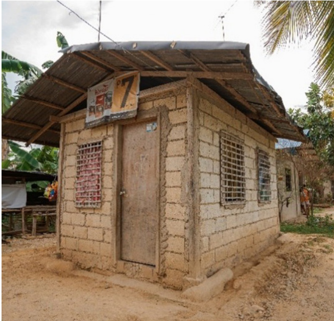
This home in the Philippines was built without a strong foundation, making it particularly susceptible to disasters. Habitat's Terwilliger Center for Innovation in Shelter supported the development of a solution called Beam Monolith that reinforces foundations and helps homes withstand the region's typhoons.
