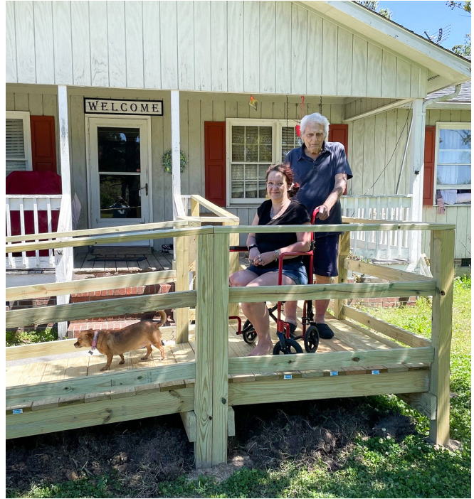
Sheila is thrilled to have a new ramp that allows her to leave her home and spend time outside.
