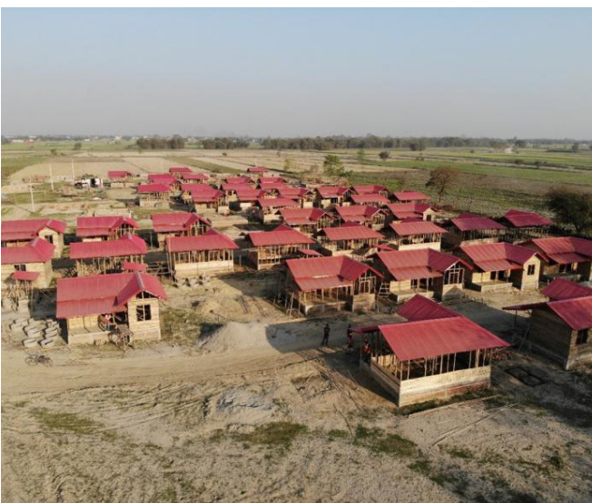
Habitat is working with local and international partners to scale cement bamboo frame technology in Nepal, with the goal of creating a self-sustaining industry to build resilient homes like these.
